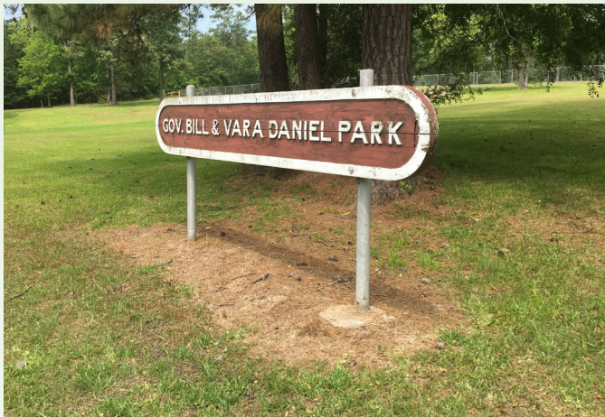
Backfill and grade around park sign to prevent further erosion and undermining.
